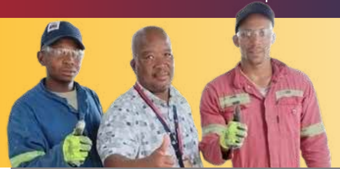
Thumbs-up from Pule Mohajane (Safety Officer) to Kagiso Matjomane and Jasel Rakolotja for wearing the correct PPE while safely chipping out broken tiles at North Decline.
